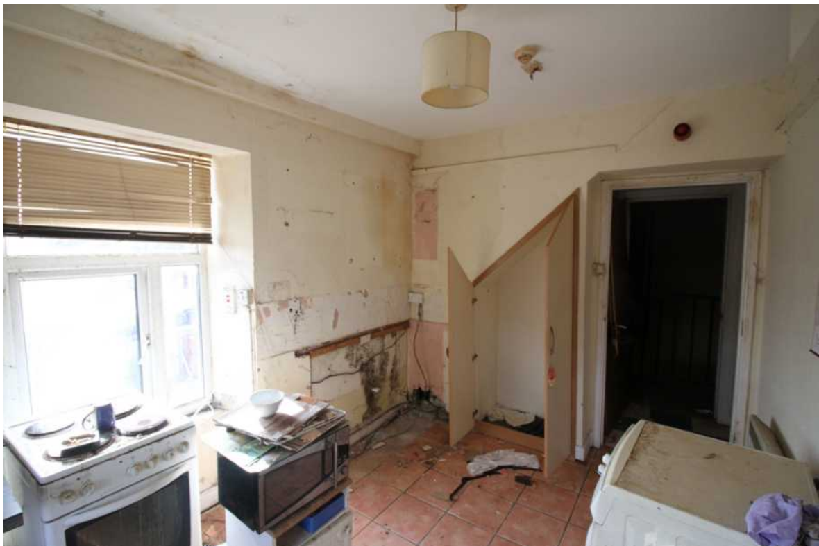
• Fig 43. Typical kitchen and evidence of damp/ mould in corners.
