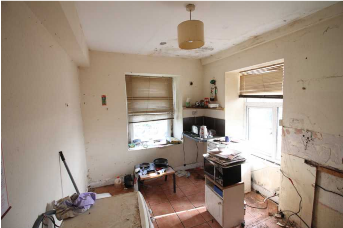
• Fig 42. Typical kitchen and evidence of damp/ mould in corners.
