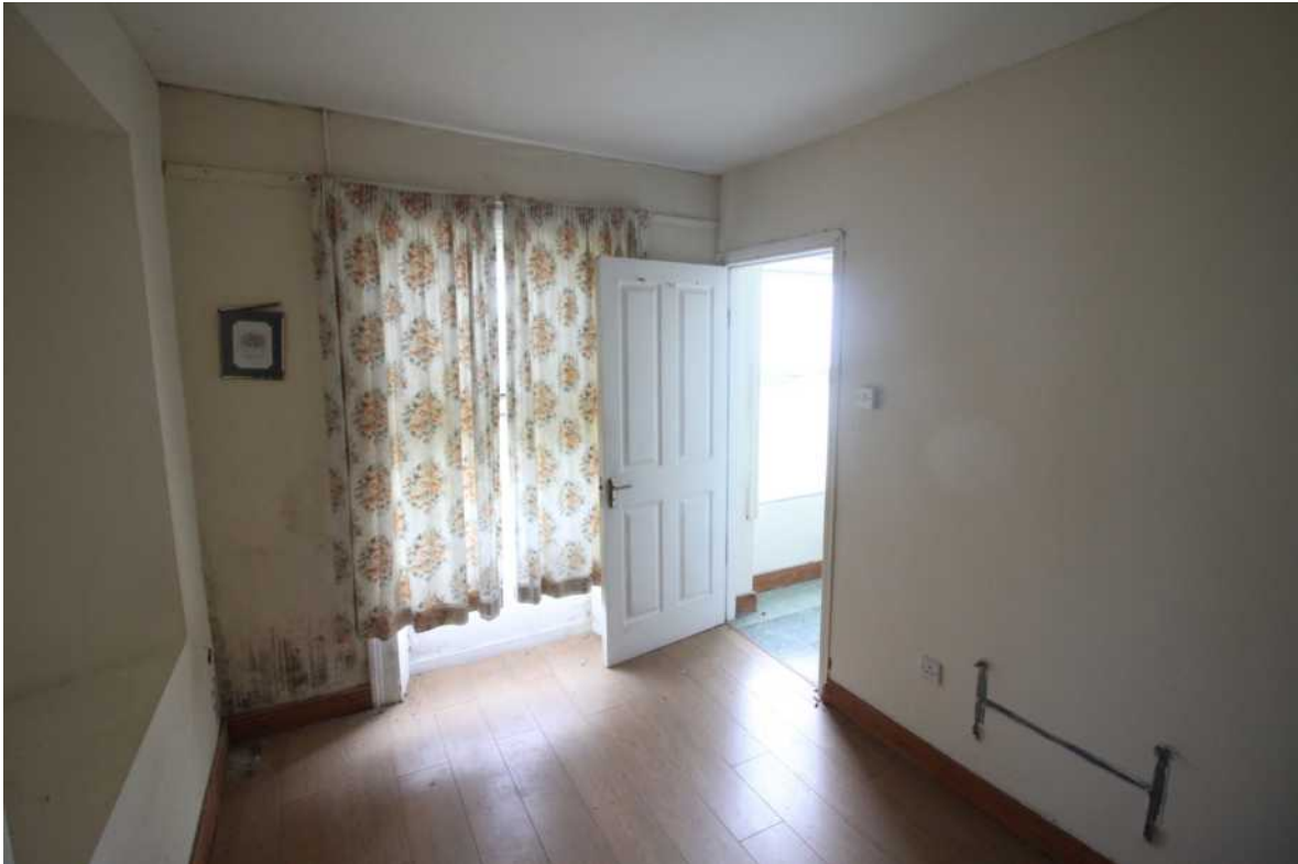
• Fig 42. Bedroom and evidence of rising damp/ mould on external walls.
