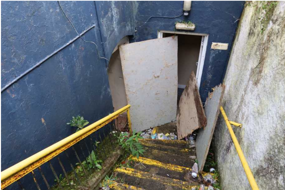
• Fig 25. Doors LGF1 & LGF 2 Lower ground floor South end two apartment entrances.
