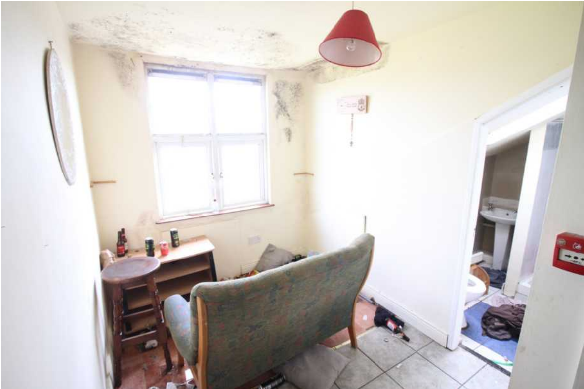
• Fig 45. Living room with damp and mould under flat roof/ at external wall.
