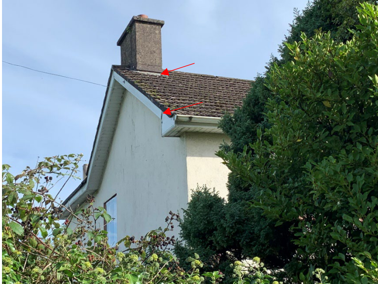
Plate 3-3: Potential access points via raised chimney flashing and a gap in the barge board on the western elevation
